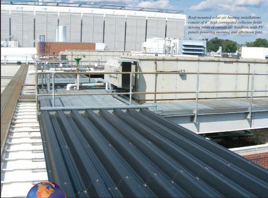
Before installation, the white walls of generator enclosures inefficiently reflected solar heat. Now, the flush panel solar siding heats air that is blown into the enclosure, and electric heating energy is reduced (l).
