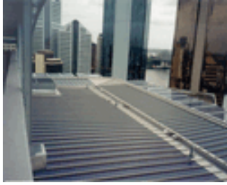
PV Laminate on Standing Seam Metal Roof
