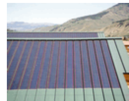
PV Laminate on Standing Seam Metal Roof
